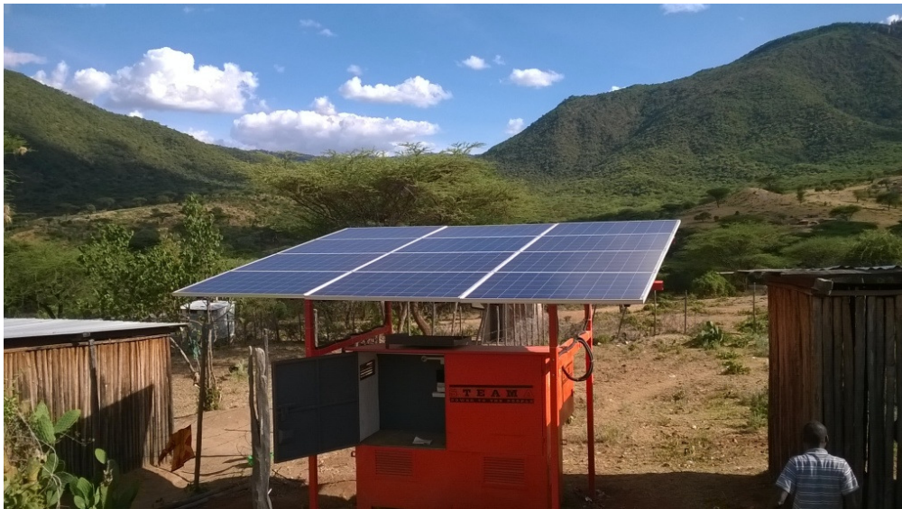
Figure 21: PowerGen project in Samburu County, Kenya showing a 3kW micro-grid
