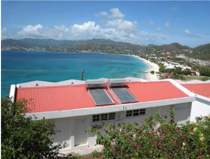
Solar Water Heaters installed on Flamboyant Hotel, Grenada
