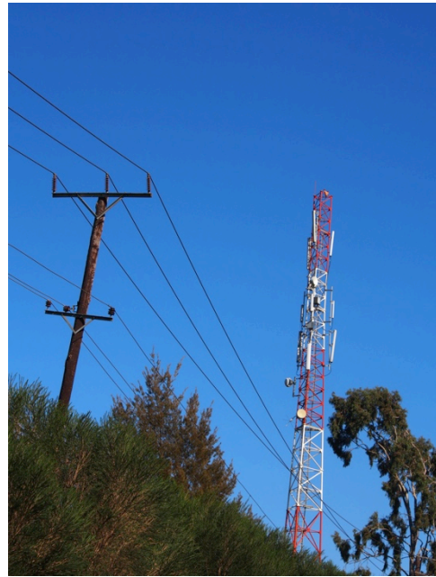
Fig. 21. Power and mobile communication infrastructure in Western Kenya
