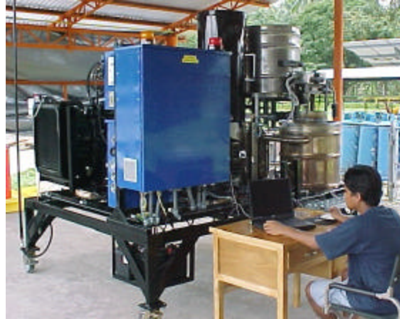
Figure 1: 15 kW BioMax power system fueled by locally available coconut shells
