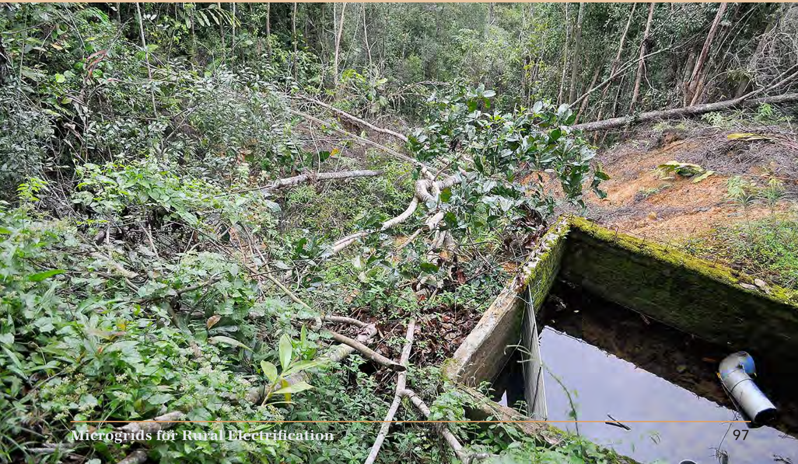
Landslide that destroyed GE/T/P microhydro penstock and forebay in Sabah, Malaysia
