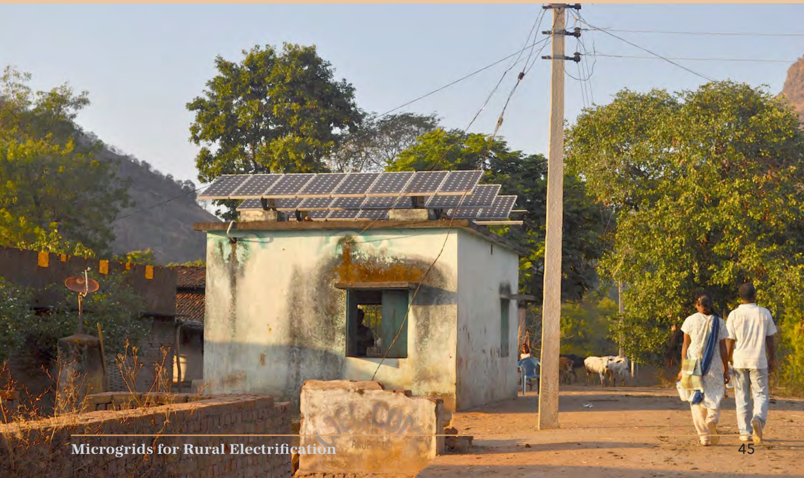
Solar PV array at an OREDA microgrid site in Orissa, India
