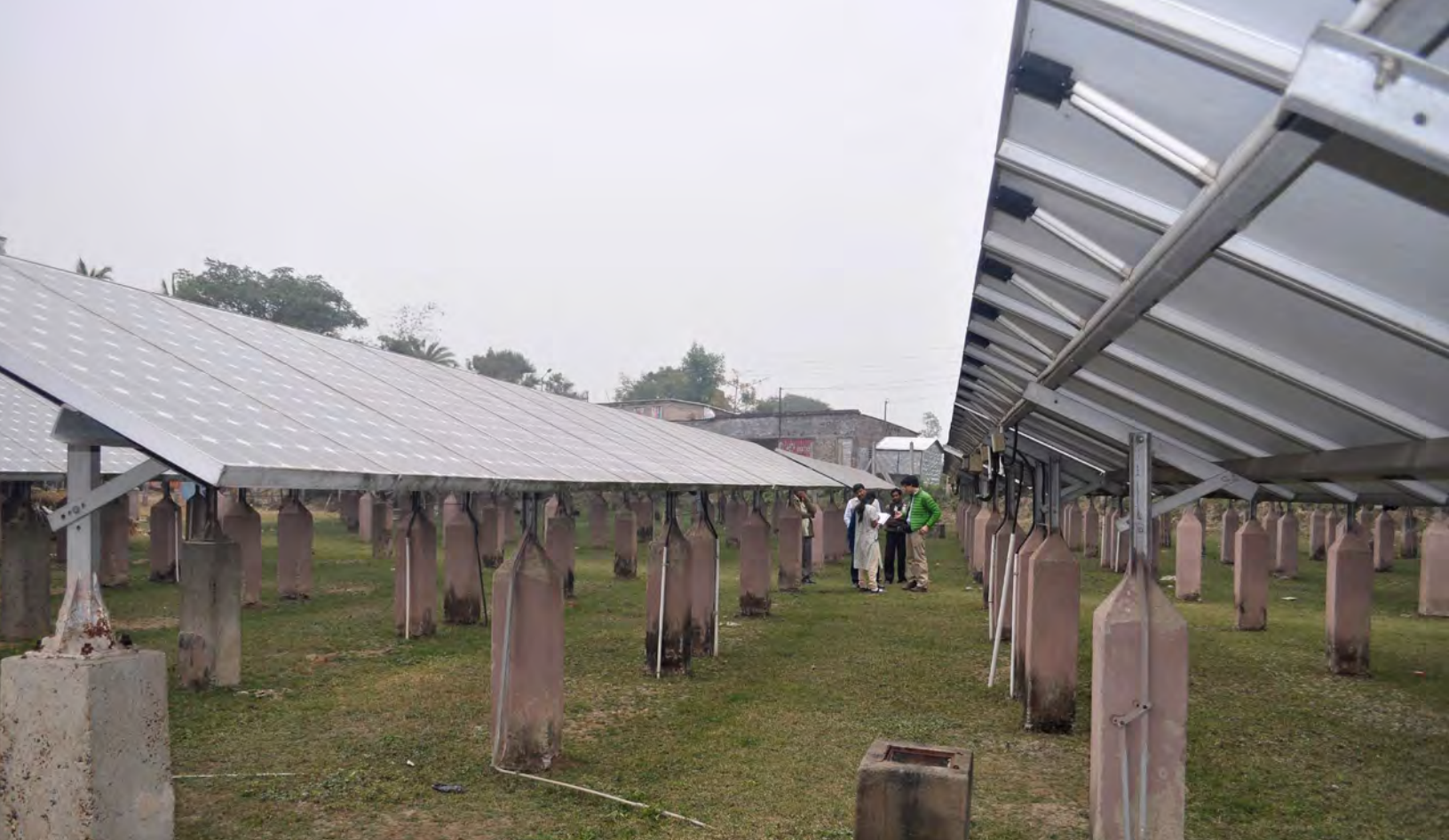
A glimpse of the 120 kWp solar PV array at a WBREDA microgrid site on Sagar Island, India
