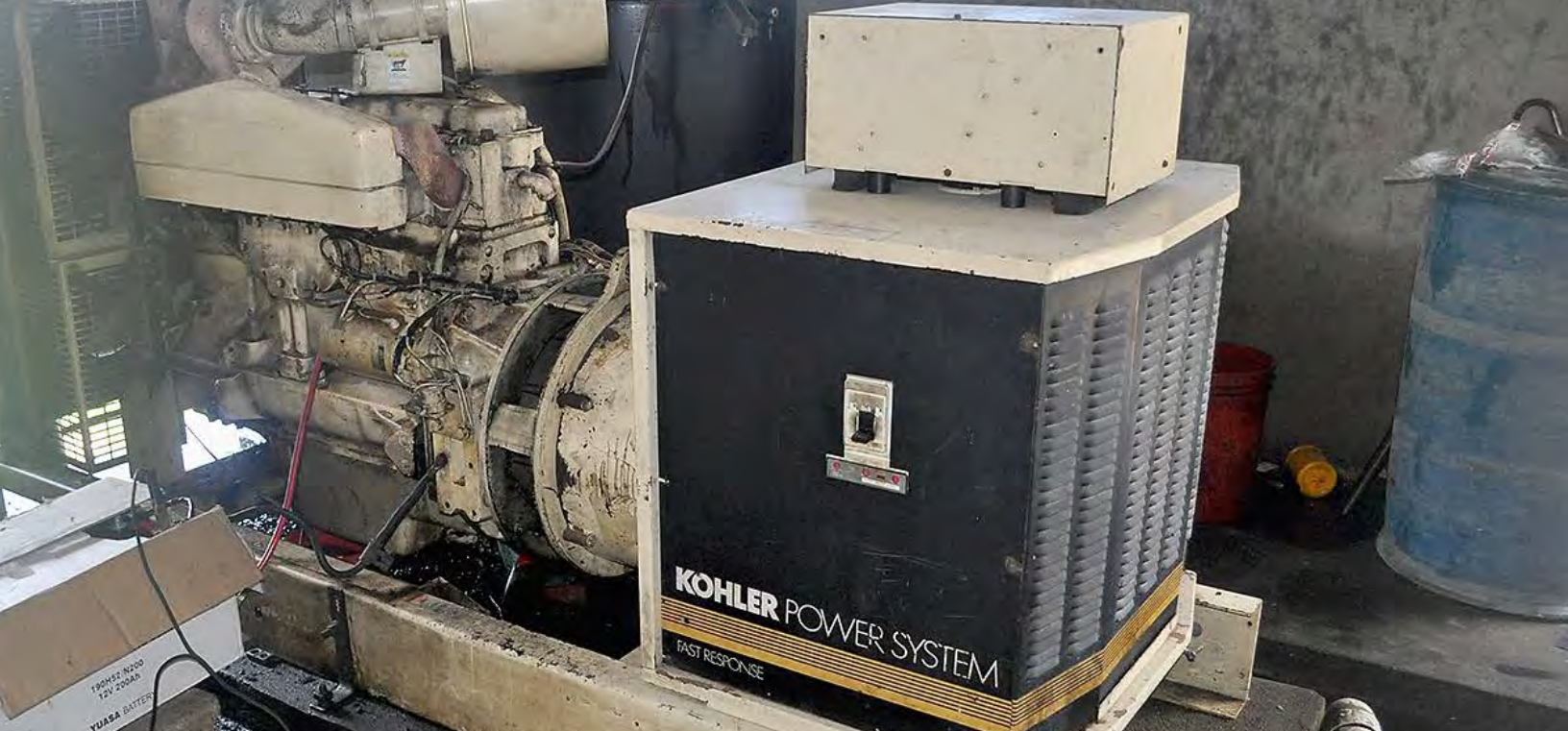
Diesel generator in need of repair that powers the Coteaux microgrid in Haiti, built in 1994
