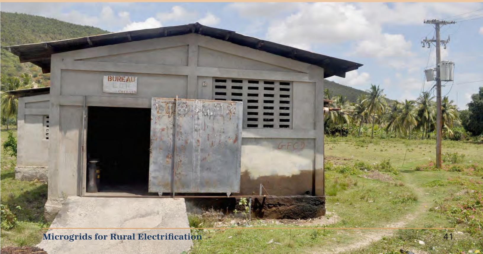
The generator house and step-up transformers at the Coteaux microgrid in Haiti
