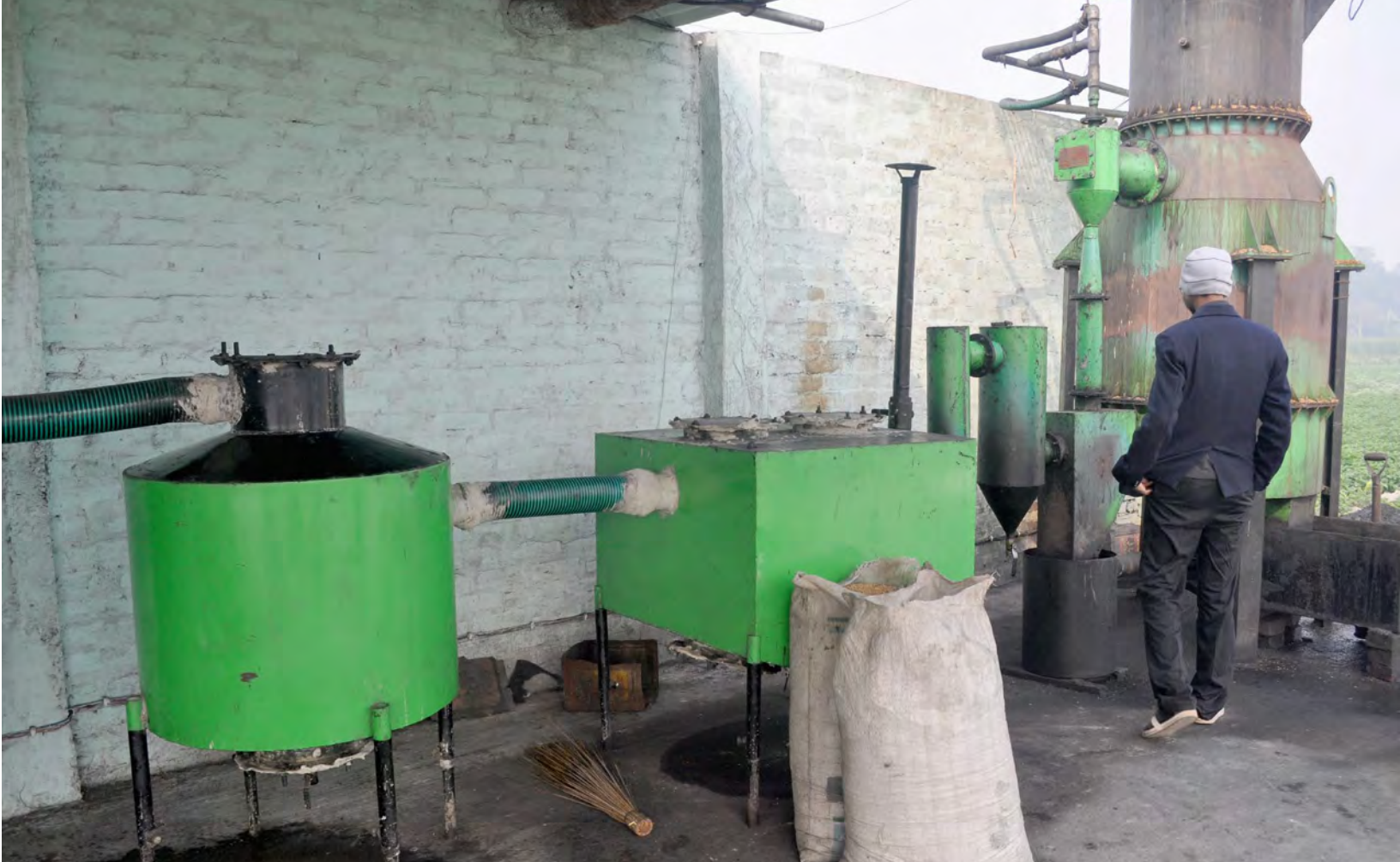
A biomass gasifier plant at a HPS microgrid site in Bihar, India
